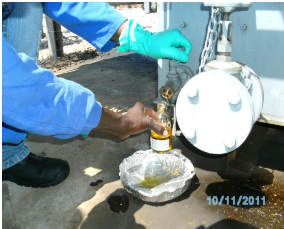
Figure 6: A seasoned worker handling transformer oil with bare hands
