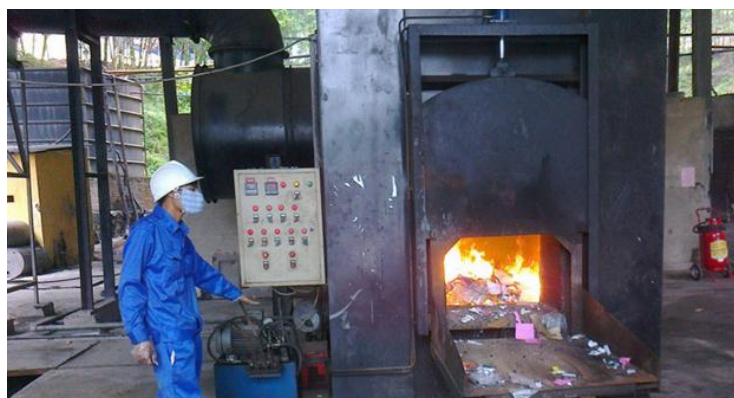
Figure 21. A hazardous waste incinerator made in Vietnam
