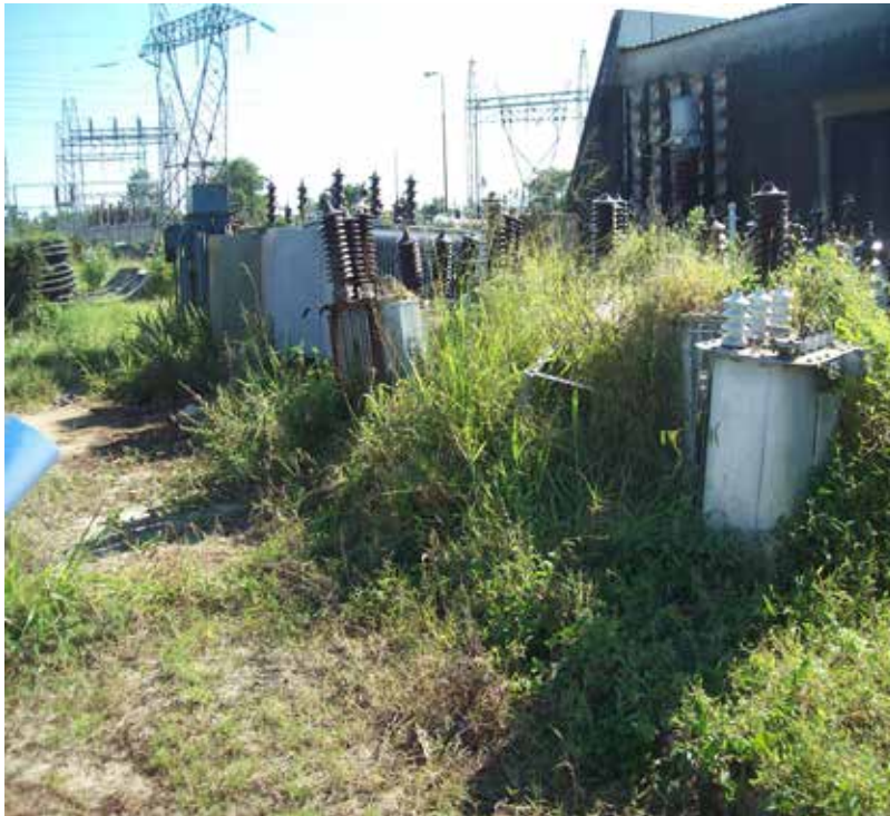
Figure 9: Old Transformer at Mtoni Power Station
