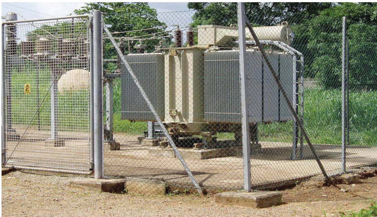
Figure 5: Main transformer receiving current from source - Bo
