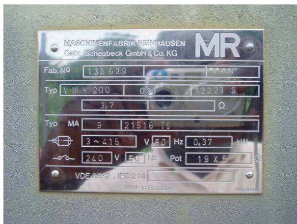
Figure 7: Transformer name plate in Bo-Kenema
