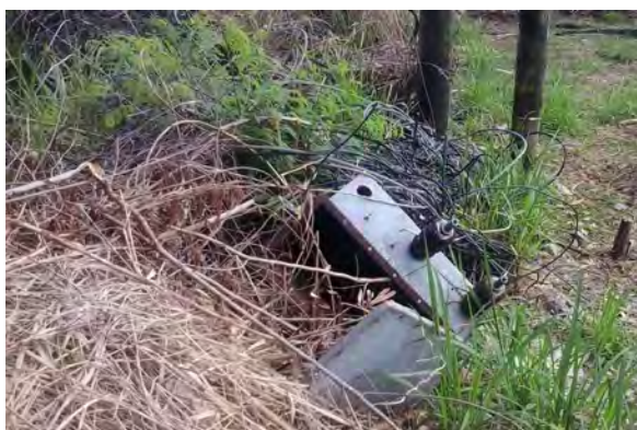
Before March 2014: Empty transformer dumped at ex PUC waste oil stockpile (PCB)
