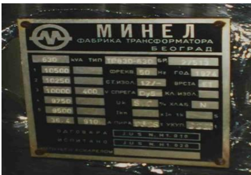
Figure 2.3.3.1.2.c: Nameplate on transformer produced in Serbia
