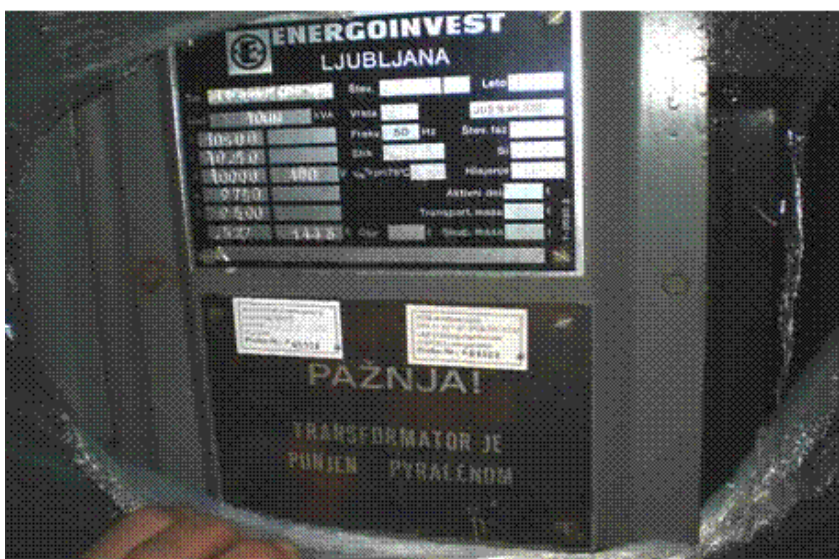
Figure 2.3.3.1.2.b: Nameplate on imported transformer
