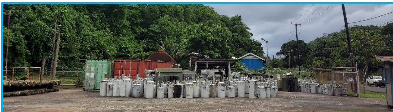
Figure 2-6: Obsolete transformers in storage at LUCELEC's Union Compound
