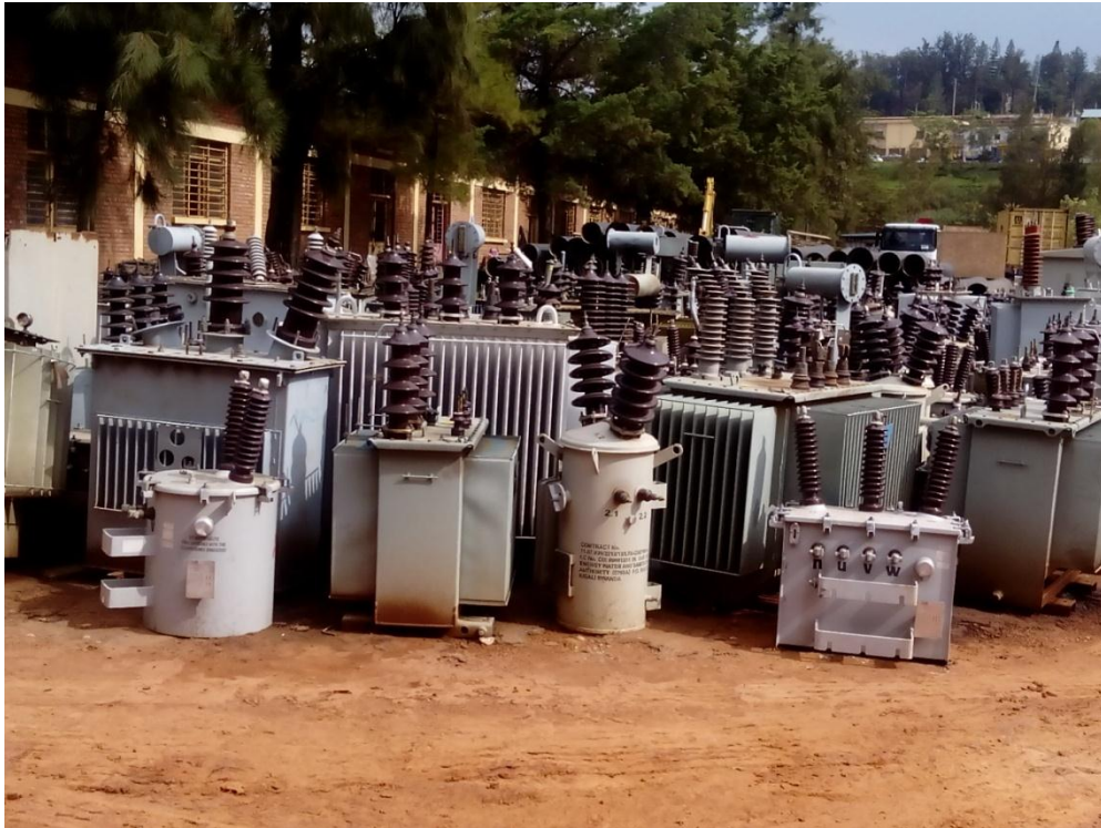
Figure 3: Is showing malfunctioning transformers stored at REG repairing workshop also used as temporary storage area at Gikondo central store.
