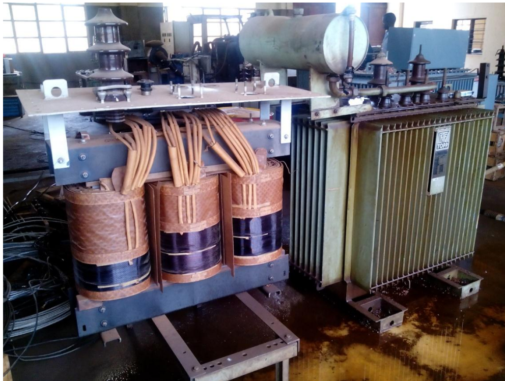
Figure 2: Is showing malfunctioning transformers at REG repairing workshop at Gikondo central store.
