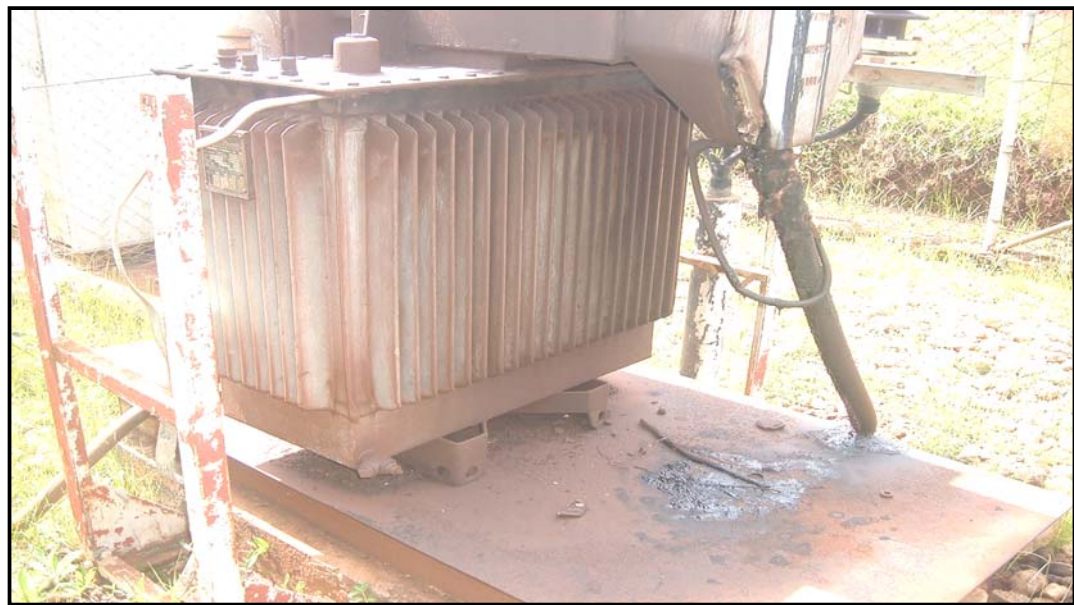
Photo 3: Plate support and ground contaminated below the transformer of 75 KVA (year 1955) in the South of Butare Airstrip
