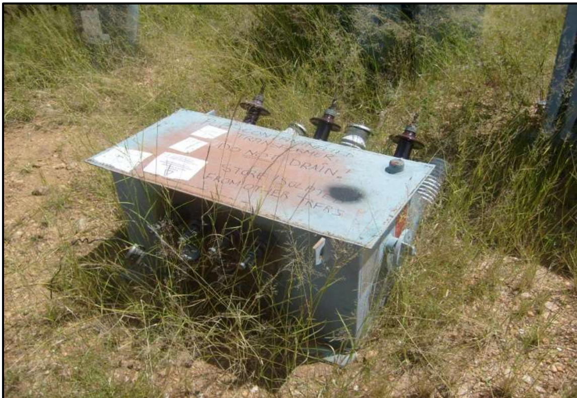
Figure 6 showing transformer storage at Brakwater (Source: NamPower, 2014)
