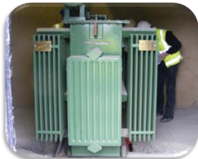
Inspection of an Electrical Transformer
