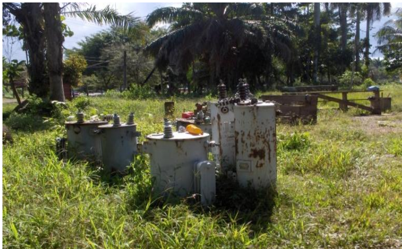
Figura No 14. Transformers in the open air.
