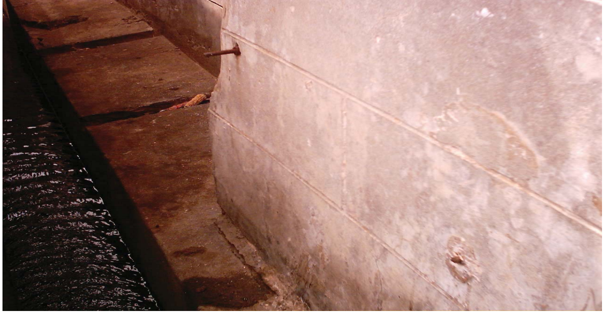
Plate 3: Drains around repair building choked with black contents of transformers
