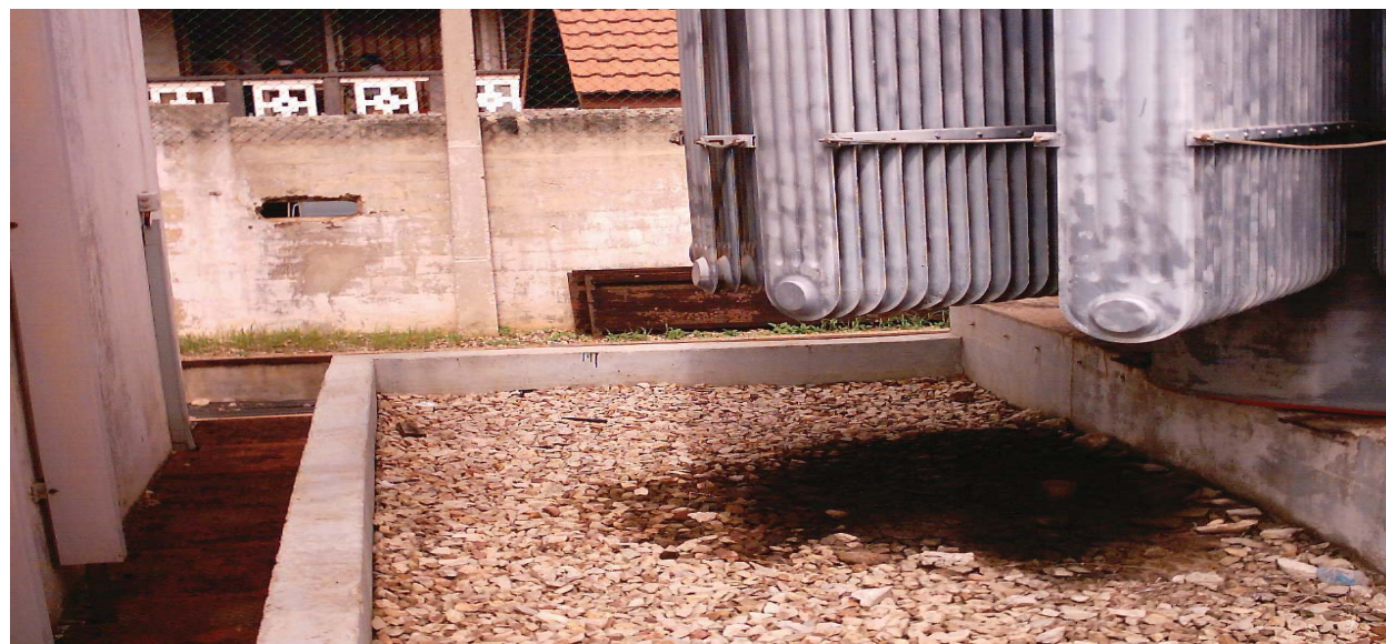
Plate 1: A contaminated site: Immediate environ of a transformer contaminated by spillage
