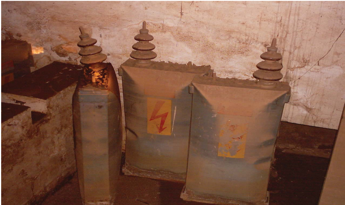
PLATE 6: CAPACITORS BROKEN AT THE INSULATOR END OR BULGING OUT ON THE SIDES
