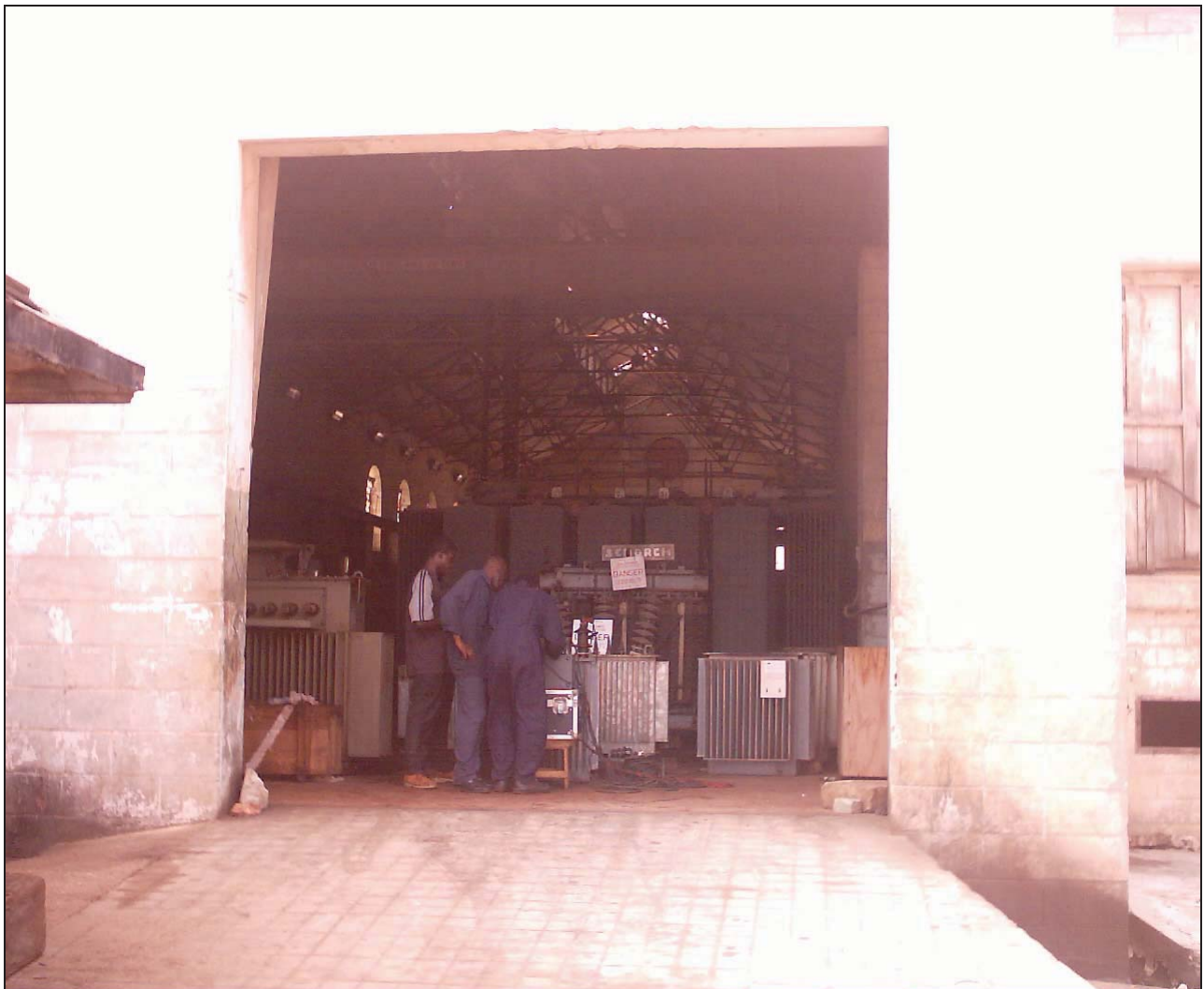
Plate 2: Technicians of the Electricity Company of Ghana at work in the transformer repair building
