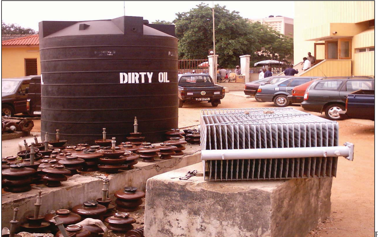
Plate 4: Displayed reservoir for PCB/oil waste at the Accra Central Power Station G
