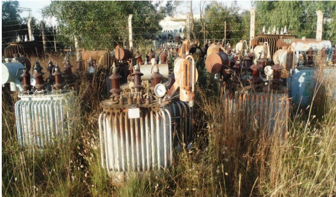
Figure 5: Some of the PCB oil containing old transformers
