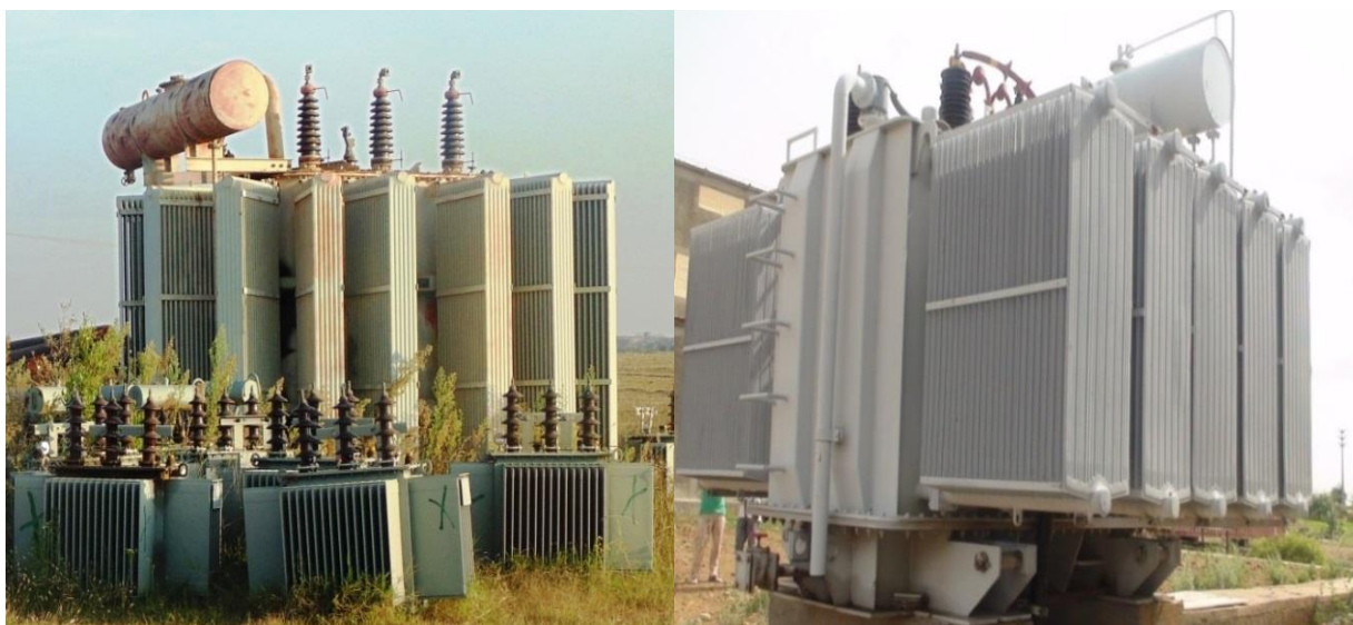
Figure 6: Representative PCB free transformers in use in the country
