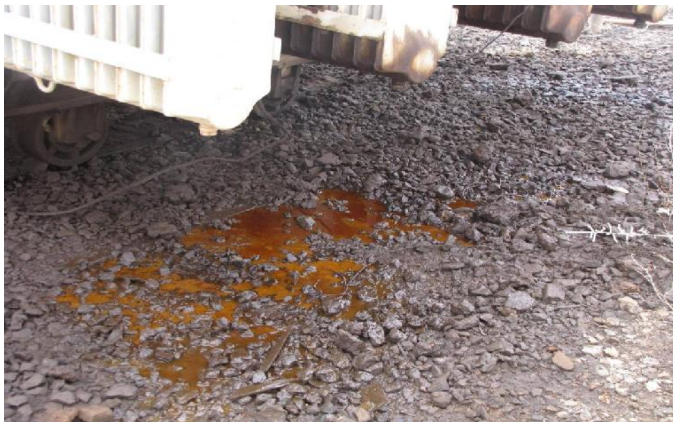
Contaminated area in Girar Power plant
