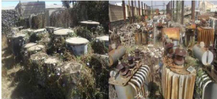
Above, Denden and Girar substation decommissioned transformers
