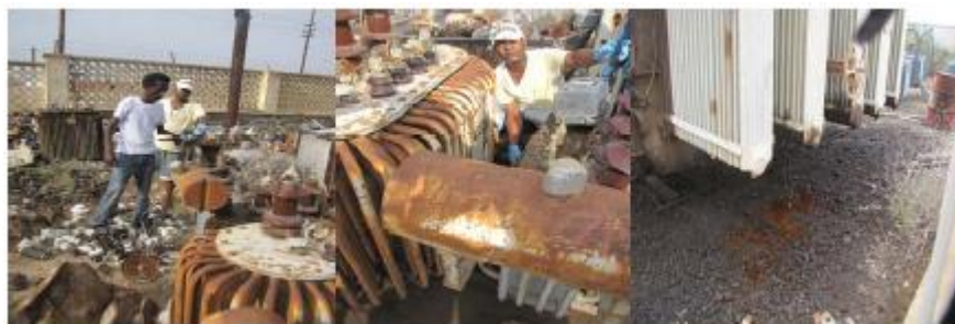
Taking samples and reading plate on Girar substation by PCB task teams and contaminated soil in Girar substation.
