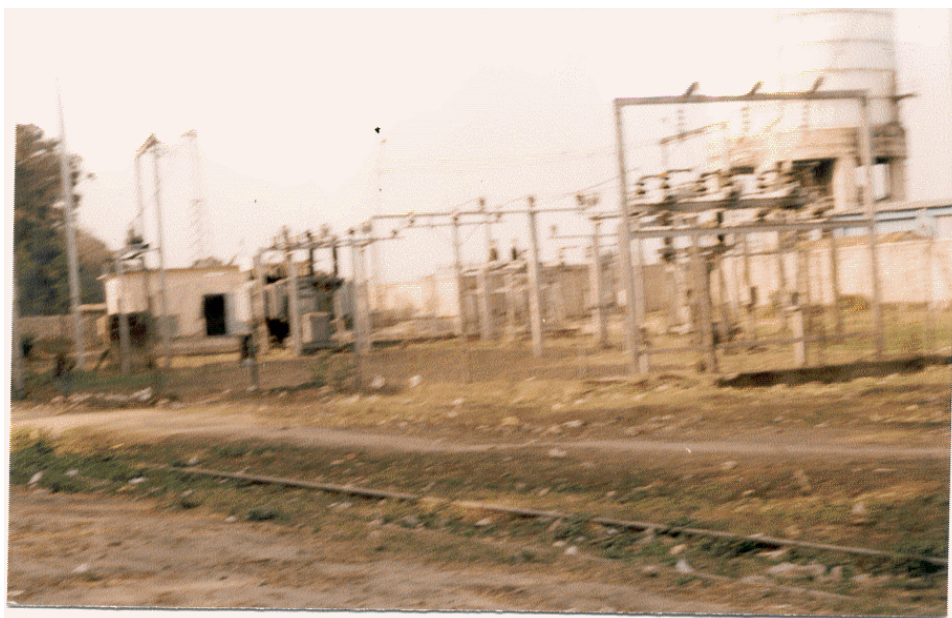
Figure 10: Transformer station in Moukoundzi Ngouaka (Brazzaville)
