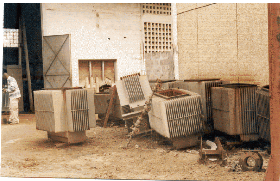
Figure 11: Decommissioned transformers at SNE Headquarters in Pointe-Noire
