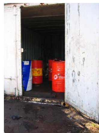
Image 10: PCB oil storage at Moroni power station
