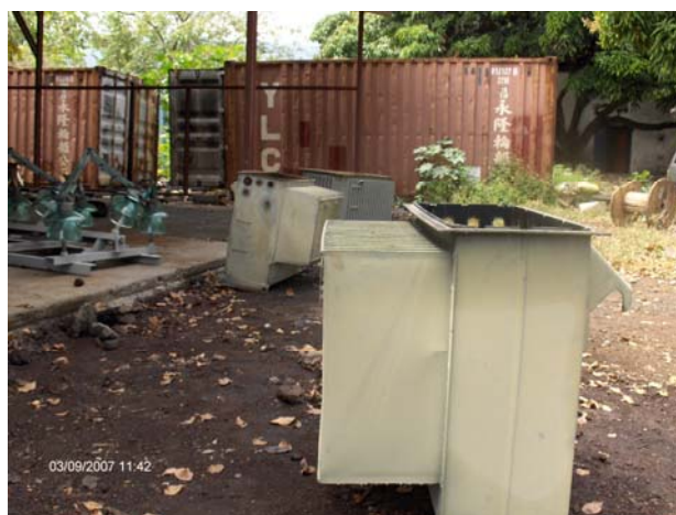
Image 8: Open storage of transformers, MAMWE's electrical facility in Moroni
