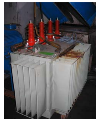
Image 7: MAMWE's decommissioned transformers located in Moroni
