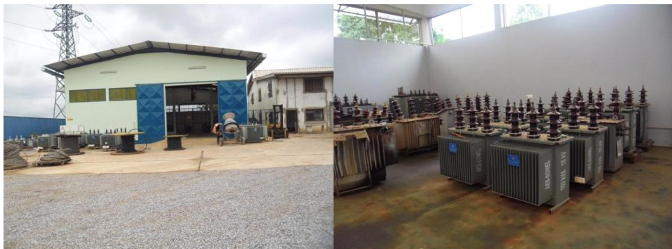
Figure 1 : Storage warehouse of transformers with PCB in Ngouso (Yaoundé)
