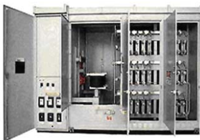
Picture 6. Power factor correction capacitors
