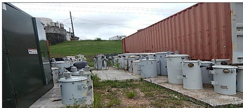
Figure 4: < 50ppm PCB Transformer stockpile at FLPC, Spanish Lookout, Cayo District.
