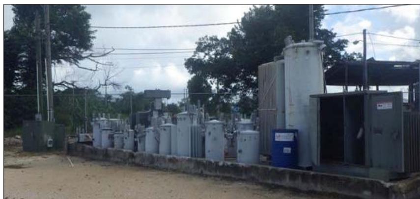
Figure 5: Stockpile of decommissioned transformers at BEL's warehouse facility in Ladyville, Belize District.
