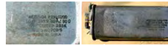
Sealed capacitors containing PCBs in high concentrations
