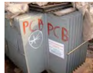
Electrical transformer containing PCB (PCB level > 500 ppm)
