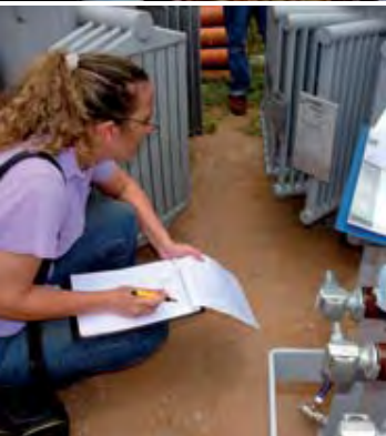
Inventory of transformers in Paraguay
