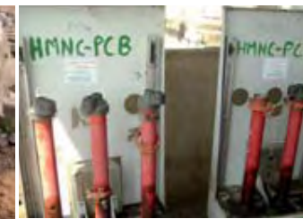
Circuit breakers containing non-contaminated mineral oil
